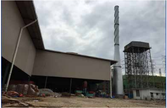
Overview of Stack & Furnace Area
