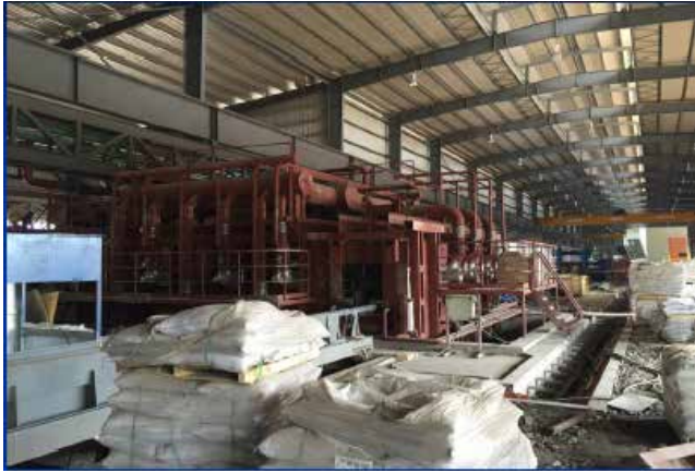
Reheating Furnace Area
